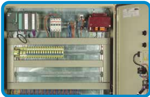
Standardized group control for normal systems and central control for complex waste disposal
