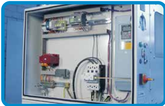
Clear arrangement of all electrical and control components
