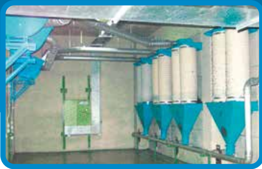
Disposal of waste from DHC or / and A/C filter dust collectors
